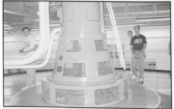
V-8ers saw the entire workings of a power dam, including the internal turbines, generators, and the control room.
